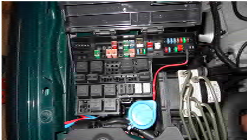
2 x relays (R9/R10) shown light grey. Harnesses for these can be seen lower left of fuse box. DRL live feed connected via Piggy Back fuse connector F38 (live on ignition) A slot has to be cut in lid to allow for Red Wire.
