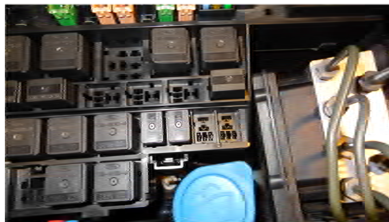
Showing relay bases R9/R10 after loading with cables. (I was going to fit the DRL Control 5 pin relay to R15 - but that was very difficult to access so opted for external mounting)
