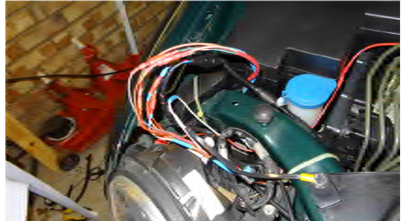
Showing all connections to relays and fuse box. (Note GROUND wire connected to radiator top mount bolt)
